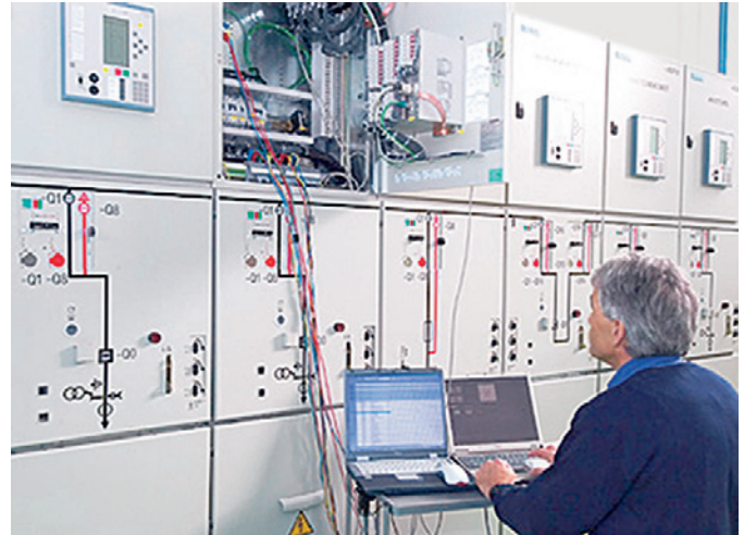
Fig. 2/34 Protection engineer at work
