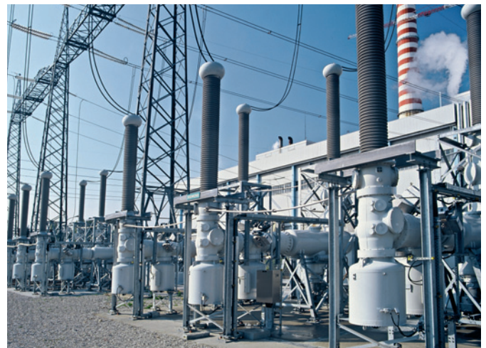
Fig. 2/10 Application in the high-voltage system
